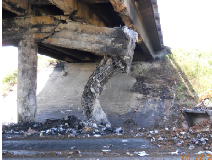
Figure 1.2. Damage caused by the tractor-trailer collision with the SC Highway 150 bridge over I-85 (Smoke 2012)
