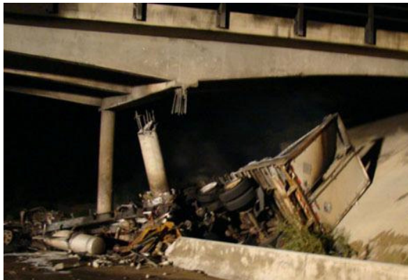
Figure 1.1. Road 26.5 pier support failure caused by tractor-trailer impact in Grand Junction, CO (Gallegos and McPhee 2007)
