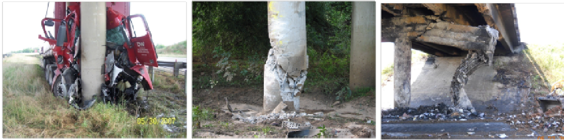
(a) (Buth et al. 2010) (b) (Buth et al. 2010) (c) (Smoke et al. 2012) Figure 6.40. Examples for (a) minor, (b) major, and (c) extensive damage states
